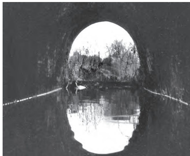
Looking east out of the California portal in 1961. Photo from Edwin Fasham, Lapal Canal Trust
